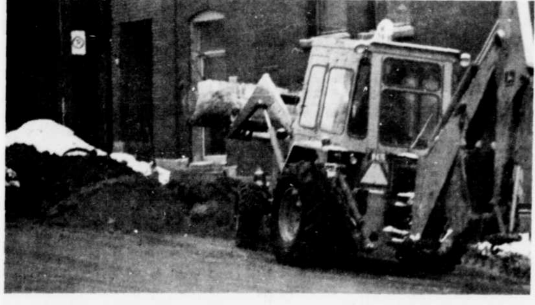
DIGGING UP — The unseasonal weather we have been experiencing recently has created havoc in many areas of the city, including sewers and underground pipes. The city's trusty employees are always busy digging and filling. (Record photo service)
