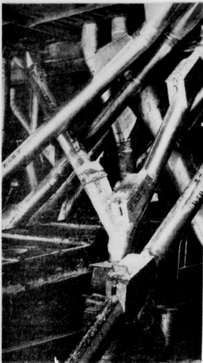
PLUMBER'S NIGHTMARE? — No, this is simply the aspiration duct-work in the Carey Canadian mill which directs the flow of air to the filters.
