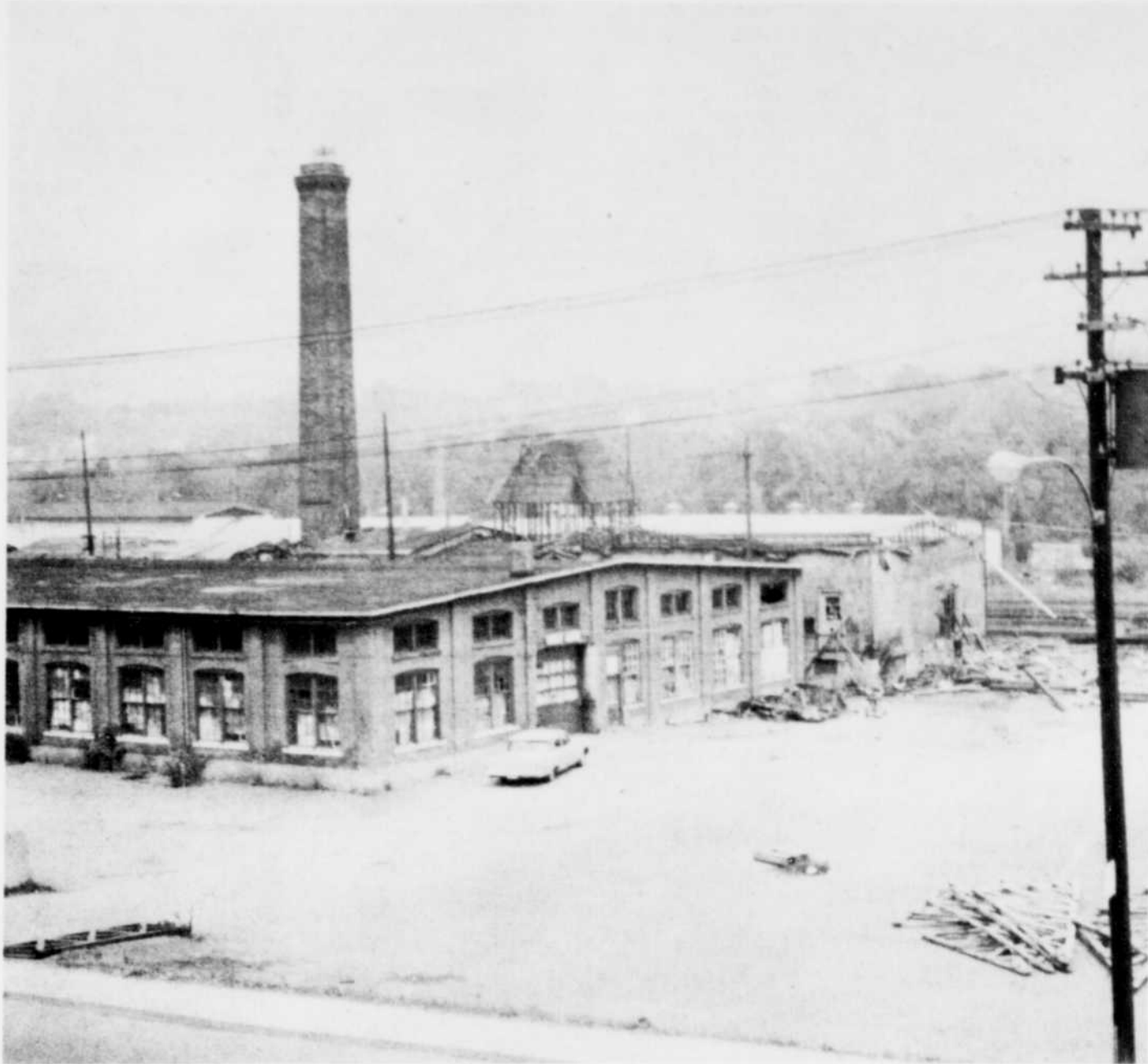
WHAT NEXT? — Workers are busy demolishing the L. O. Noel buildings on Wellington Street South this week to make way for a future construction site. A high ranking official at Denault Ltd., large scale grocer suppliers, said recently the company
