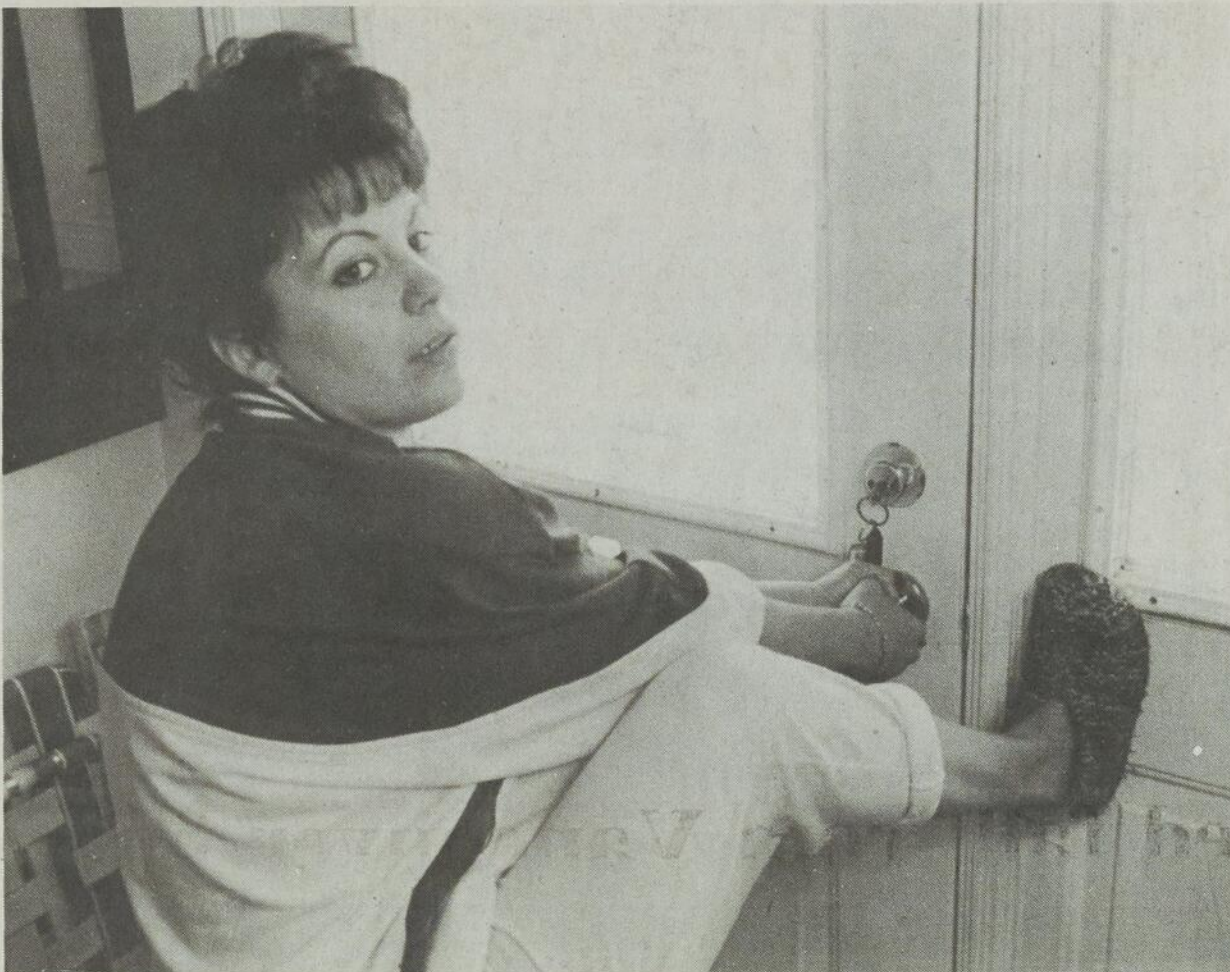
Sylvie St-Jean has to brace herself to open her ill-fitting front door. The builder has repeatedly ignored requests to fix the problem.
