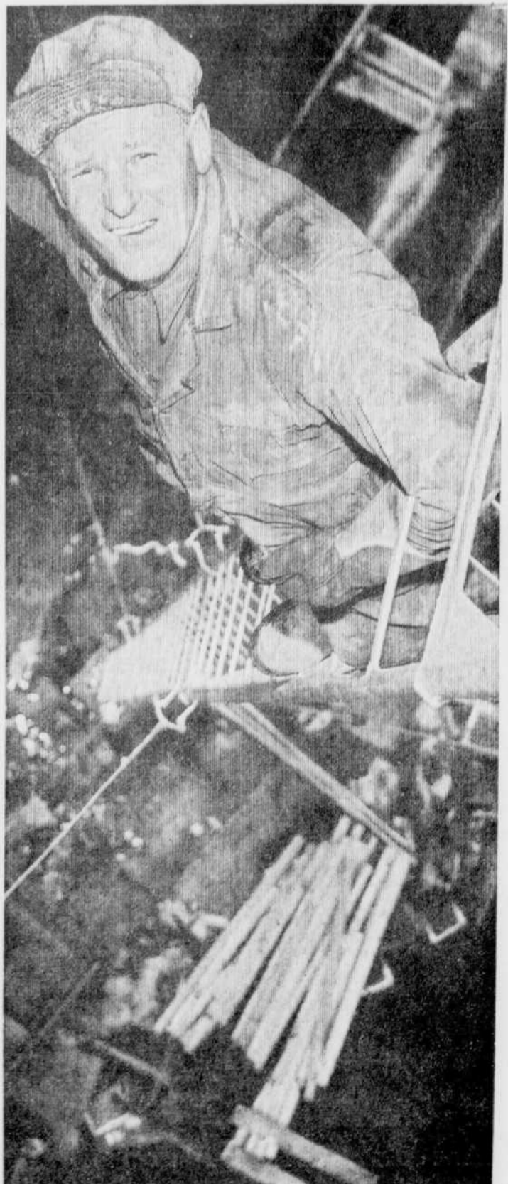
RISKY REWARDS — Steeplejack Joe Lachance climbs up a 180-foot radio broadcasting tower on Lulu Island, near Vancouver. Such risky jobs earn the Quebec-born 53-year-old veteran at least $100 a day. His work on high buildings, towers and bridges involves painting, construction, engineering and demolition. Some of his jobs take him 400 feet above ground. (CP Photo)
