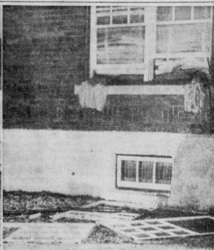
DEBRIS SCATTERED ON LAWN
