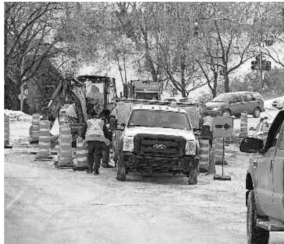
Contractors work to expose and fix a water pipe problem at the corners of Lansdowne and St. Catherine St., January 7. The tie-up caused minimal traffic problems and was repaired by the following afternoon.
