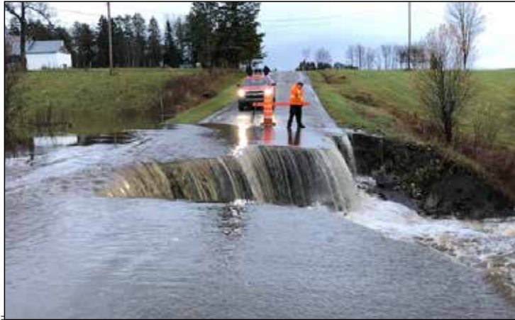
Road washout on Route 255 in 2019. (Photo: John Mackley)
