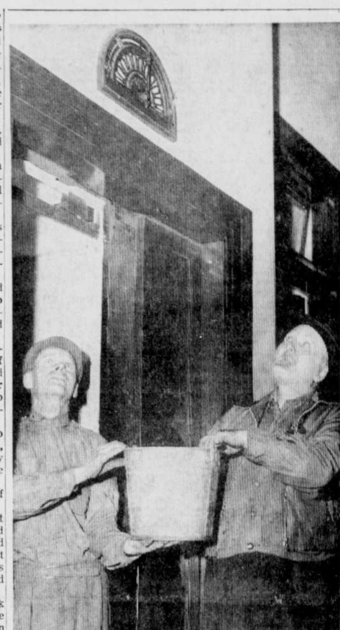
SPRING THAW — These two Sherbrooke court house employees aren't playing a game. They're catching drops of water which started to seep through a fault in the court house roof Friday and onto the floor of the main hallway. Officials say repairs to the roof are underway.
