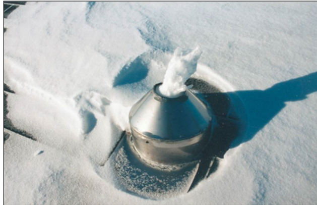
FIGURE 4.7: ICE FORMATION AT THE VENT STACK OUTLET SOURCE: SHQ
