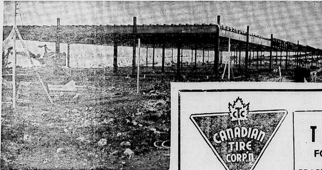
The Chateauguy Regional Shopping Plaza on D'Anjou Blvd., is now definitely showing signs of progress. Most of the steel frame, has been erected and in some places the walls are now going up. While opening date for the first stores is the beginning of May it will be several months later before the whole project has been completed.
