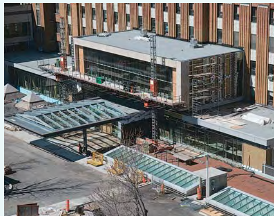
New front entrance and lobby during the final phase of construction in mid-spring.
