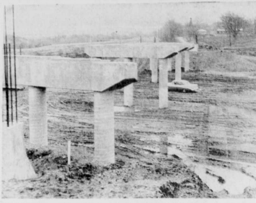
GIANT PILLARS — Pictured above are some of the huge concrete pillars that will support part of the new Vermont interstate highway, which is expected to be completed shortly. The highway will connect with the Canadian four lane highway in the east section of Rock Island and Derby Line. (Record Photo by Andre Pepin)
