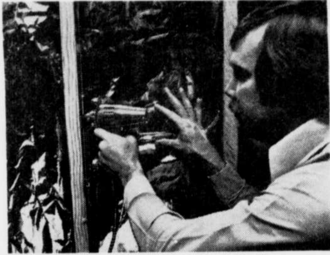
YOUR WINTER FUEL BILL will be smaller if you put up insulation now during the fall. Easy-to-handle blanket insulation and a new electric staple gun make the job simple for any do-it-yourselfer, and it saves money, too.
