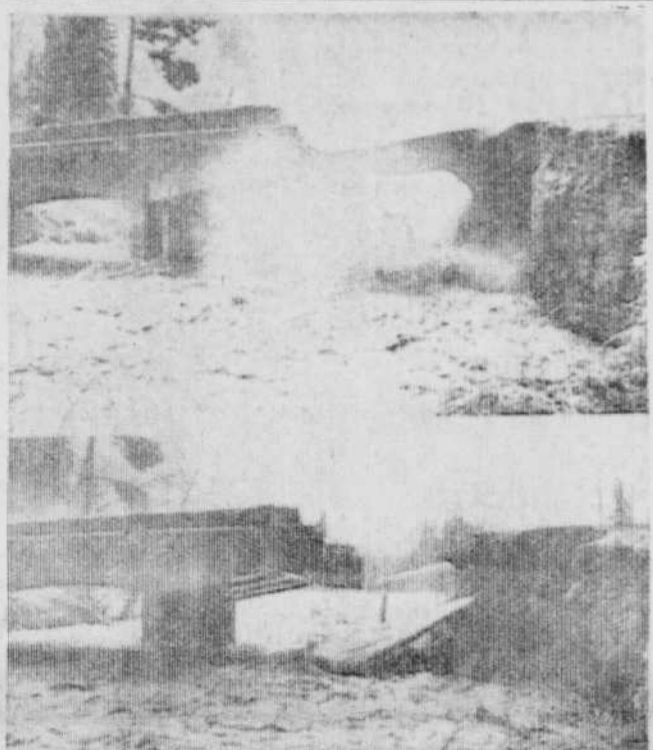
BRIDGE GOES OUT — This bridge is among many which were washed out in Oakbridge, Oregon area yesterday. Top picture shows most of roadway still connected to the bridge. Bottom shows last part of roadway as it plunges into the water. Actual bridge remained virtually undamaged but approach was completely washed out late yesterday.
