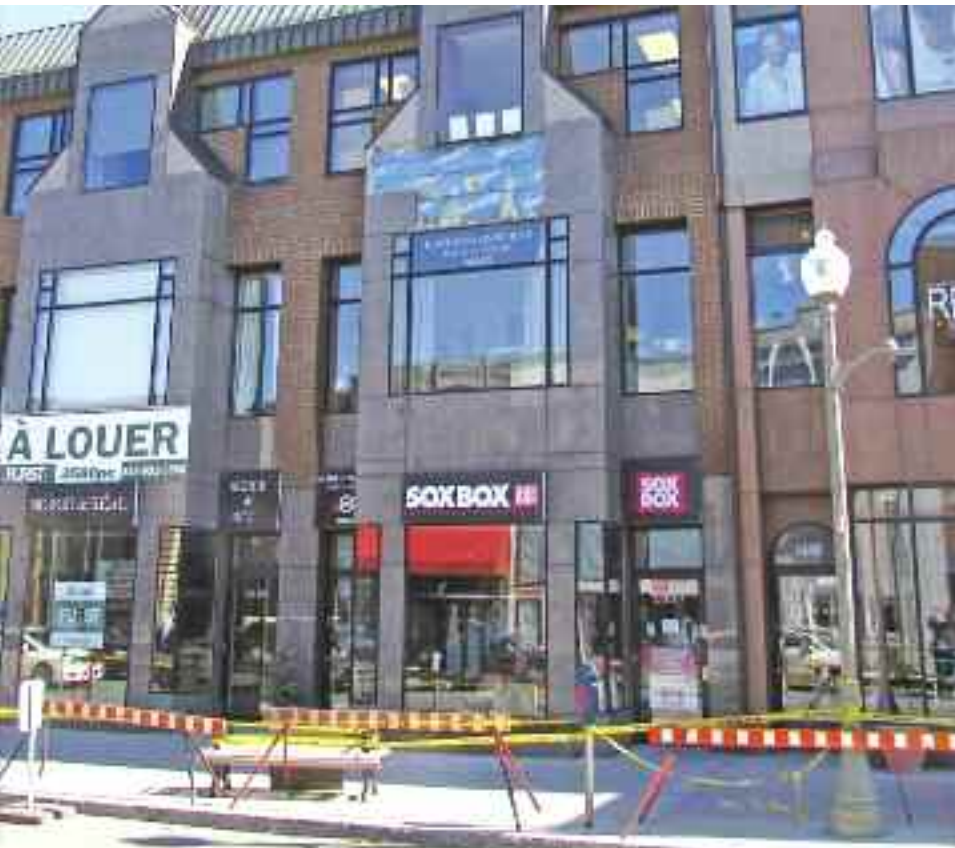
The Greene Ave. building that houses SoxBox and Kathryn Osborne Design lost some of its façade May 11. It is pictured here on May 12.
