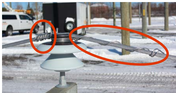
Loosened tie wires
