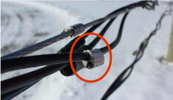
Cover missing on the connection
