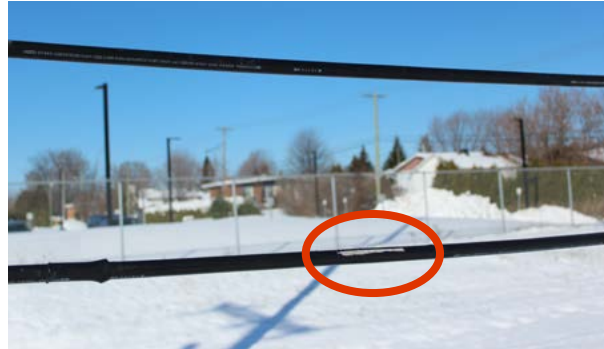
Damaged conductor sheath
