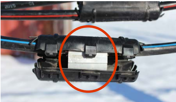
Open or damaged cover
