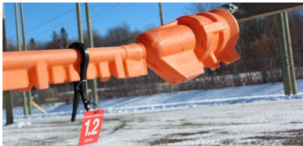
Correctly installed conductor covers
