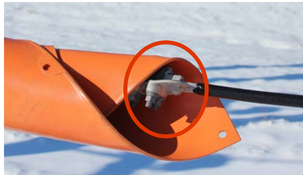
Part of the conductor is exposed
