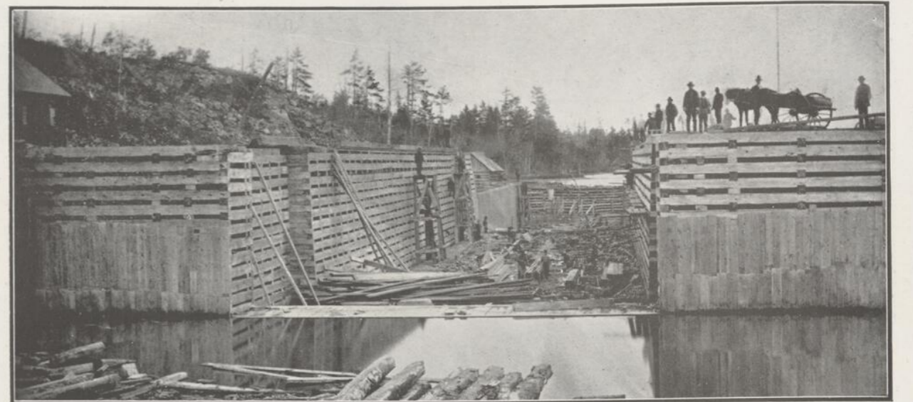
SCENES ALONG ROUTE OF GEORGIAN BAY CANAL, CANADA'S NEXT GREAT NATIONAL UNDERTAKING—View of wooden lock in course of construction, over thirty years ago, on the Upper Ottawa River, and used by steamers towing lumber. (Photograph by McLaughlin, Ottawa.)
