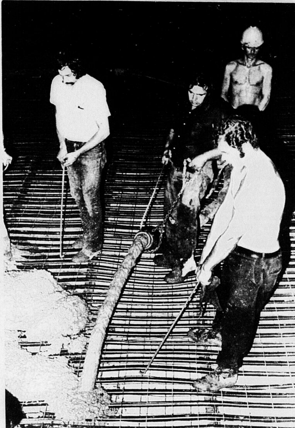
Work was carried out Monday to prepare a cement surface in the regional arena on Fairview Road in Huntingdon. The surface, designed to support an artificial ice rink, will serve a dual purpose. Activities such as square dancing and bingo during the upcoming Huntingdon Fair will be held in the building.
