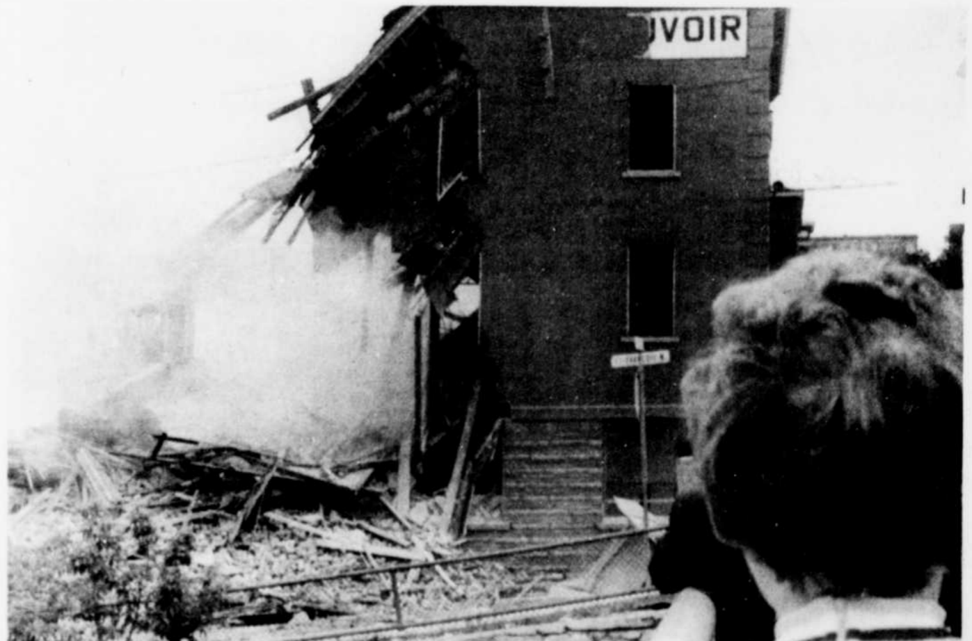
LANDMARK DISAPPEARS — One of Sherbrooke's oldest landmarks, the Belleveue Hotel at the corner of King East and St. Francis Streets, fell to the wrecker's hammer yesterday, providing a free show for passers-by. Traffic was rerouted
