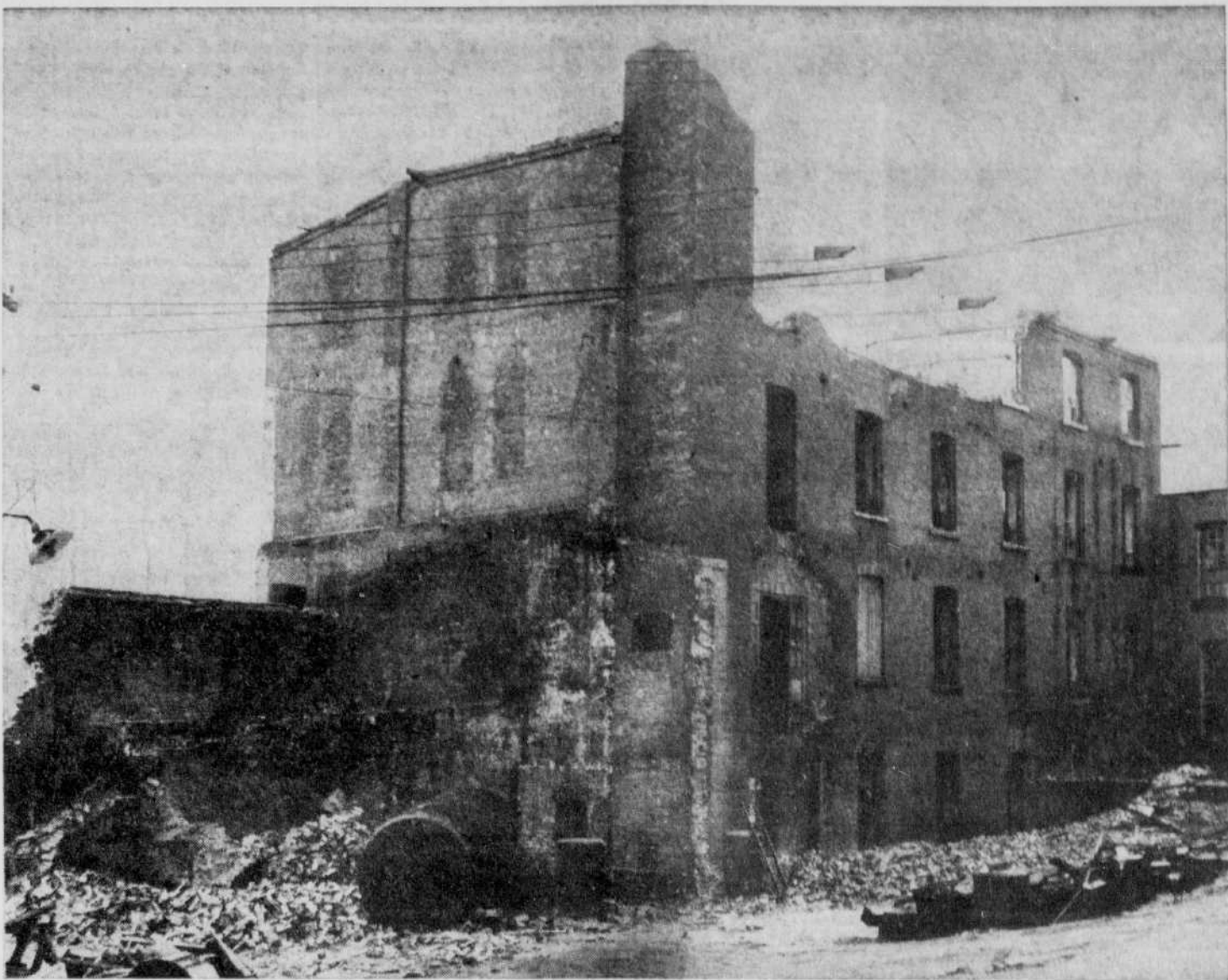
Factory Landmark Going — Once the pride of Sherbrooke's factory district which was then located along the banks of the Magog river from the Belvedere street bridge to the junction of the St. Francis, this city-owned building on Frontenac Street is being demolished after being declared unsafe. Part of the structure once housed the plant of the Canadian Edison Co. Ltd., later transferred to Peterborough, Ont., as Canadian General Electric, later being used by the Julius Kayser and by Quebec Rayon, its last tenants. (Record Photo by Gerry Lemay)
