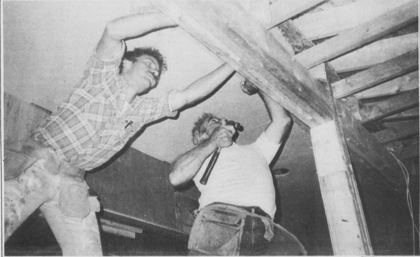
There's lots of hammering and sawing going on at the Knowlton Pub these days, but when it's over the pub should be a more inviting place than ever, with a plant-filled solarium, upstairs and downstairs bar, and meals served almost every night. The renovations were undertaken to help the legendary establishment cope with weekend crowds, and bring in more mid-week business. See our story on page 6.
