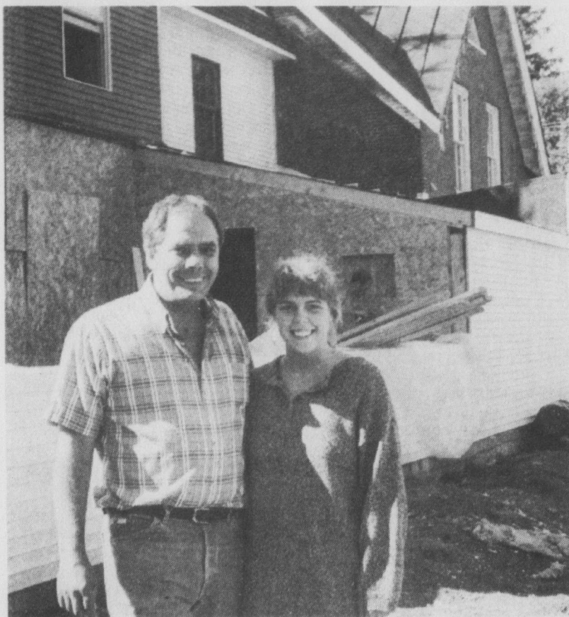
The Knowlton Pub owner Gerry Wood and his daughter Debbie are all smiles as workmen build a solarium to help accommodate the establishment's booming weekend business and encourage more visitors during the week.
