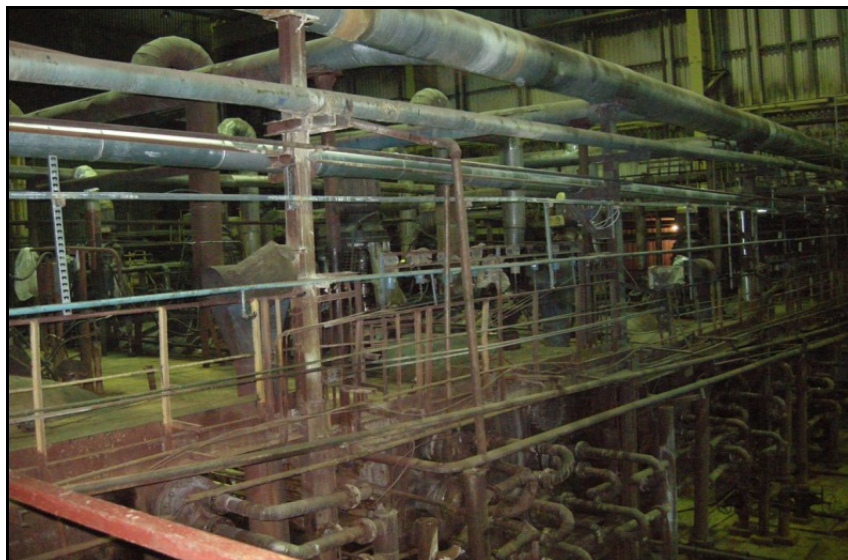
Figure 1.71: Piping to horizontal autoclaves.
