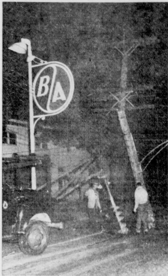
DANVILLE CRASH — A hit-and-run driver caused considerable damage when his car knocked down a power and telephone lines pole Sunday morning, on Water Street, Danville. Telephone and Power linesmen spent the night and morning in repairing the damage. Seven telephone lines were temporarily out-of-order but the power was not "cut". Two transformers were destroyed, as one fell to the ground and the other blew open. (Record Photo by Wm. H. Lunan)
