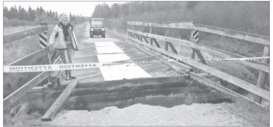
(TOURISME DES SOURCES) A cave-in along the Richmond-Danville section of the Green Route bike path has forced the closure of the section until repairs can be carried out.
