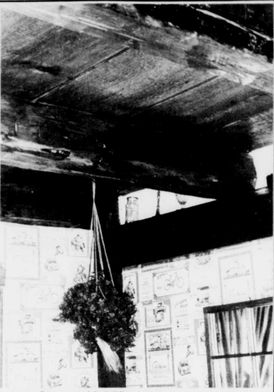
Seventy-five per cent of the buildings in Eaton Corner are over 100 years old. When residents like Marg Nicholson begin restoring their homes, they find huge hand-hewn beams like these.
