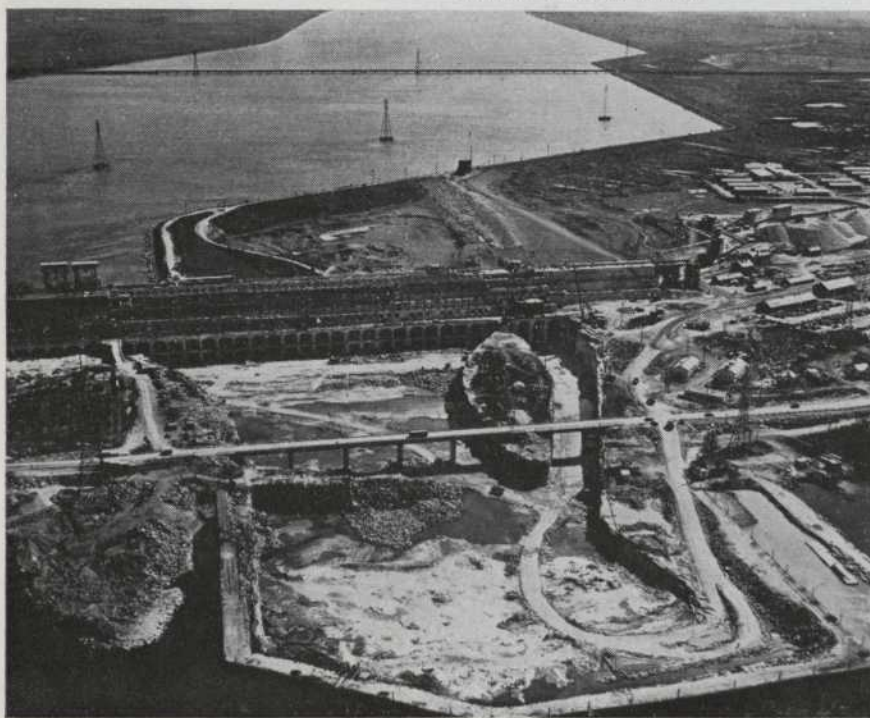
Excavation of the tailrace for the second stage development. The channel to the right of the excavation is a sluiceway through which excess water may be spilled.
