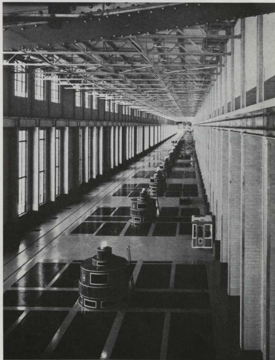
Inside view of the No. 1 and No. 2 sections of the Beauharnois development.
