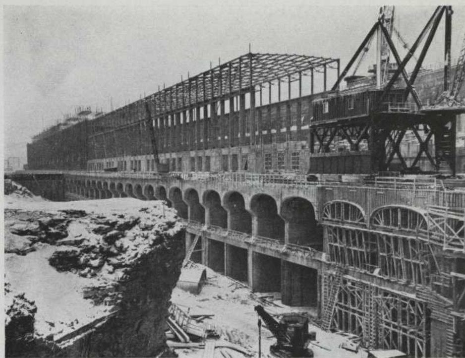
Beauharnois second phase takes shape. Beauharnois 1 at the left of the structure was in full operation when this photograph was taken.
