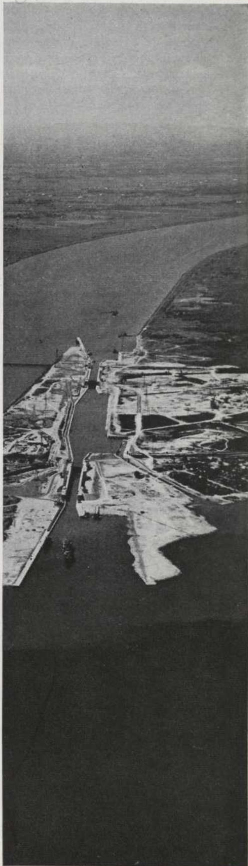
This split general view of the Beauharnois end of the power canal shows the two-fold aspect of its usefulness — navigation and hydro-electric power. On the left, the powerhouse; on the right, the seaway locks.
