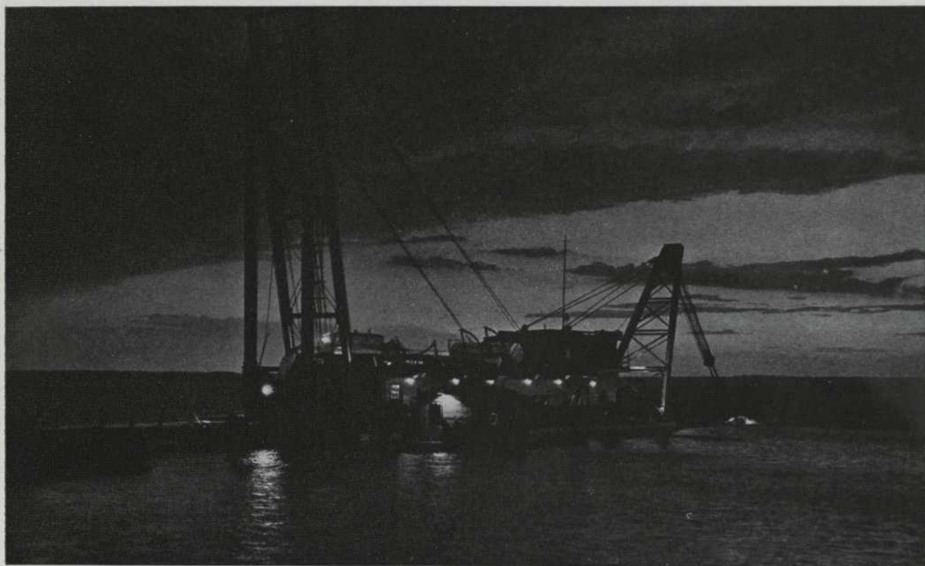
The R.O. Sweezey, one of the world's most renowned suction dredges, at work on clearing the canal as night falls. This famous dredge alone removed some 145,000,000 cubic yards from the bed of the canal.
