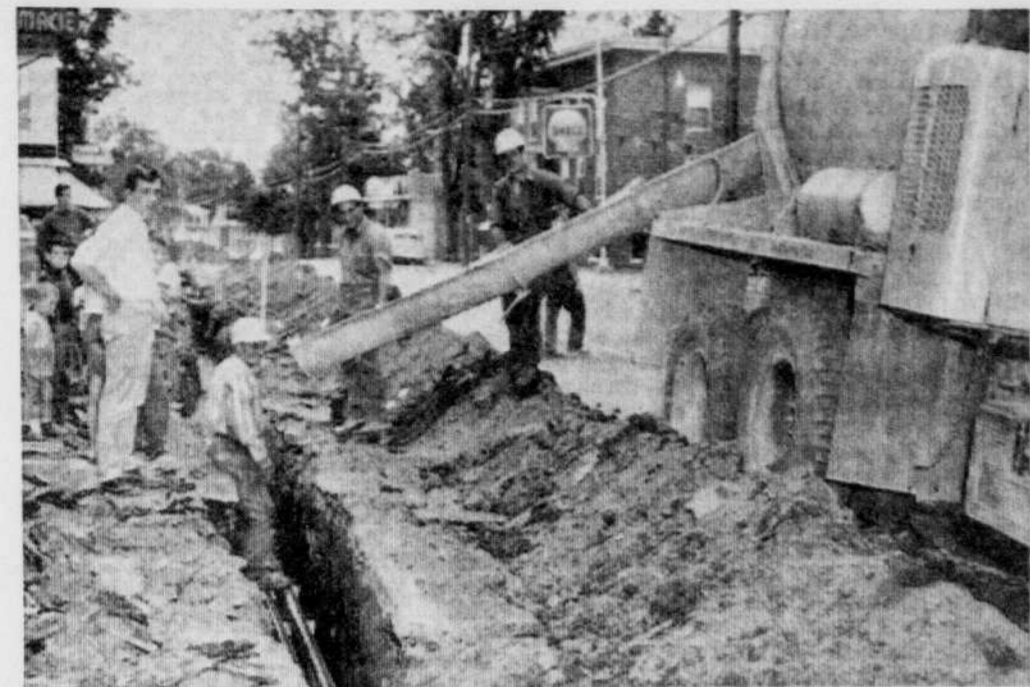
CABLE LAYING — This is a familiar scene in Cowansville as the Bell Telephone Company is laying an under-
