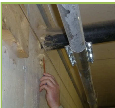
Figure 20 Smoke test done on the perimeter of a feed line sealed with foam to check for possible air infiltration
