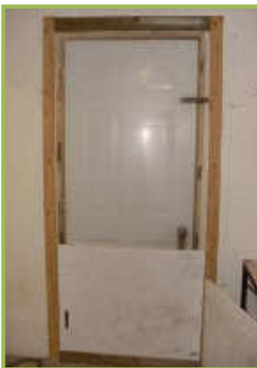
Figure 18 Door made airtight using polythene and slats around the perimeter to prevent air infiltration
