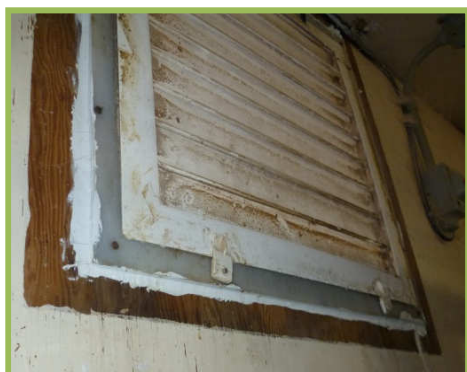
Figure 19 Perimeter of a fan housing sealed to prevent air infiltration
