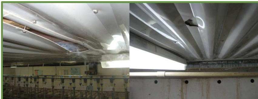
Figure 16 Breaks in corrugated plastic allowing air infiltration Photos: Darwin Reicks
