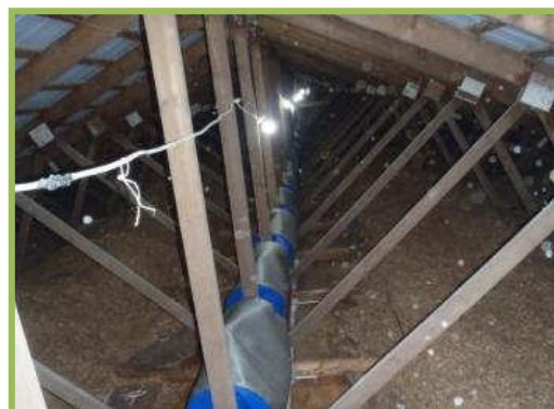
Figure 14 Dome-type antimicrobial filters installed on a continuous air inlet
