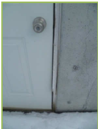
Figure 17 Non-airtight door frame lets air infiltrate and has to be replaced
