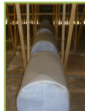
Figure 11 Dome-type antimicrobial filters with prefilters installed on modular air inlets
