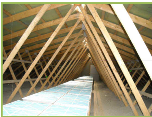
Figure 13 Mechanical filters installed on a continuous linear air inlet
