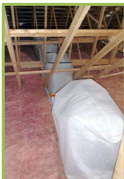
Figure 10 Cube-type antimicrobial filters installed on modular air inlets
