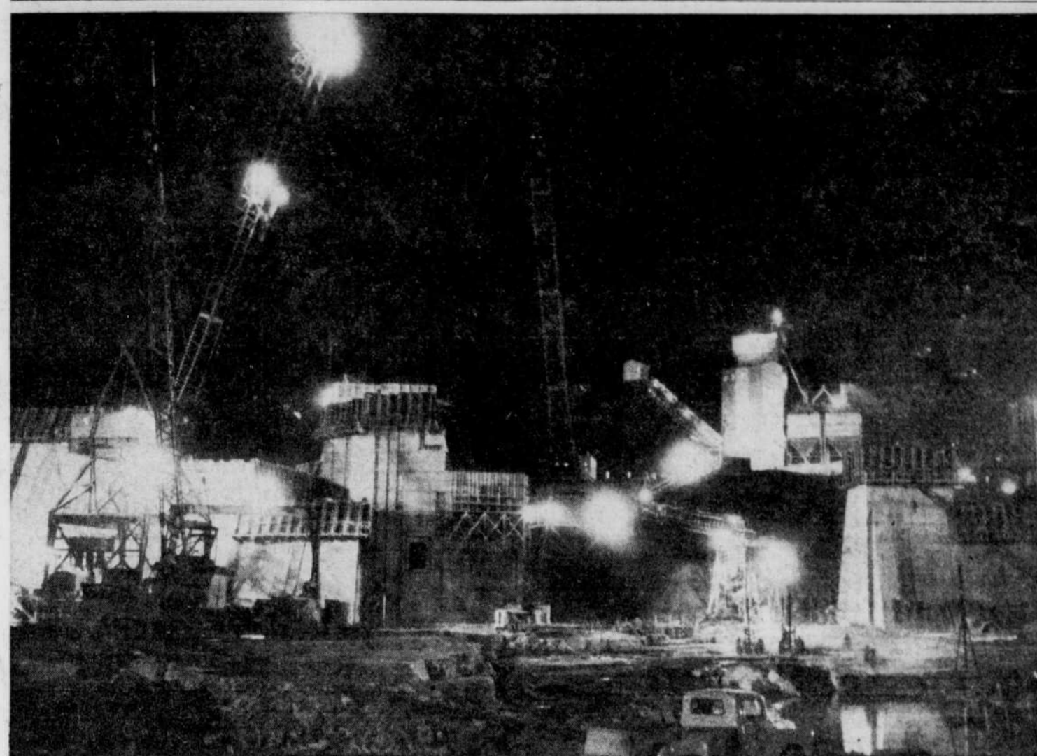
Seaway Forges Ahead and the power project of the St. Lawrence seaway is starting to take shape. This night photo shows work which goes on 24 hours a day on the Canadian end of the power house. The work is being done in the dried up bed of the St. Lawrence river and the power house will rise 162 feet from its bed rock foundation in the bed of the St. Lawrence river. Giant cement plant (top center) has already poured 26,000 cu. yds of cement in this structure, which is three months ahead of schedule. (FedNews)
