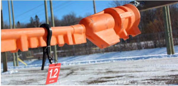
Correctly installed conductor covers
