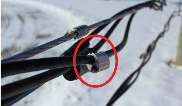
Cover missing on the connection
