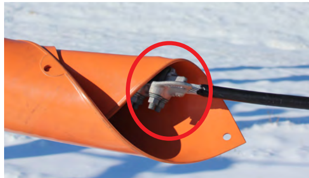
Part of the conductor is exposed
