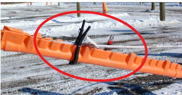
Bare conductor due to an incorrectly attached conductor cover
