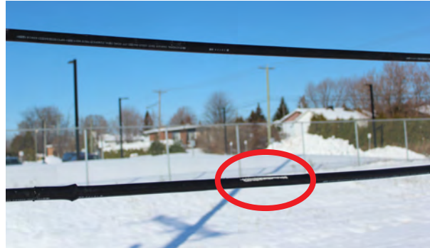
Damaged conductor sheath
