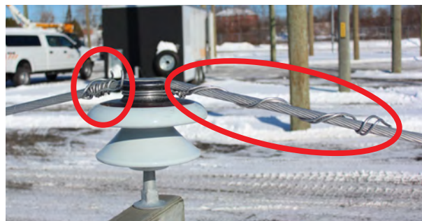
Loosened tie wires
