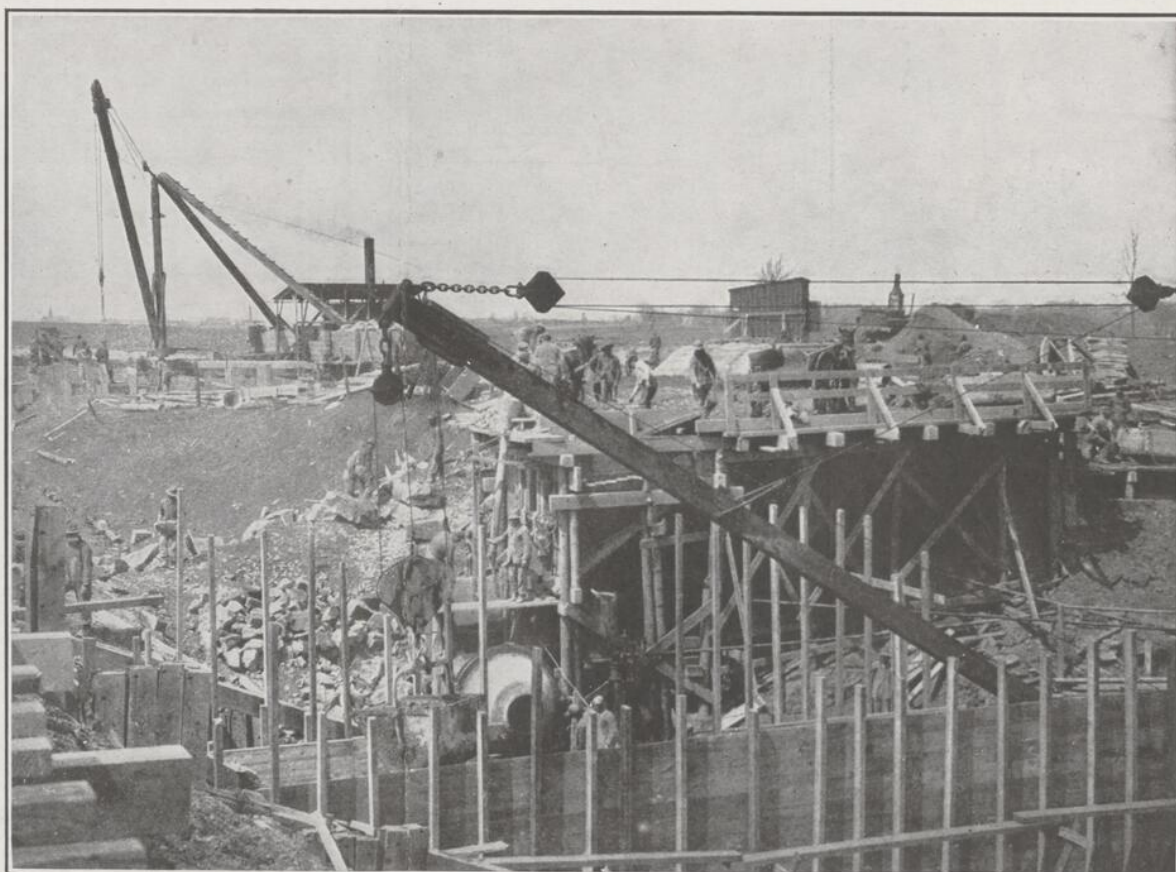
THE NEW WELAND SHIP CANAL—Crossing the present canal at lock eleven, St. Catharines. Here the two canals are at the same level.
