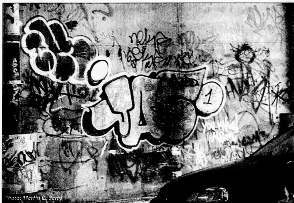
The concrete pillars beneath the Ville Marie Expressway in lower Westmount have long been a favourite target of spray-paint vandals.
