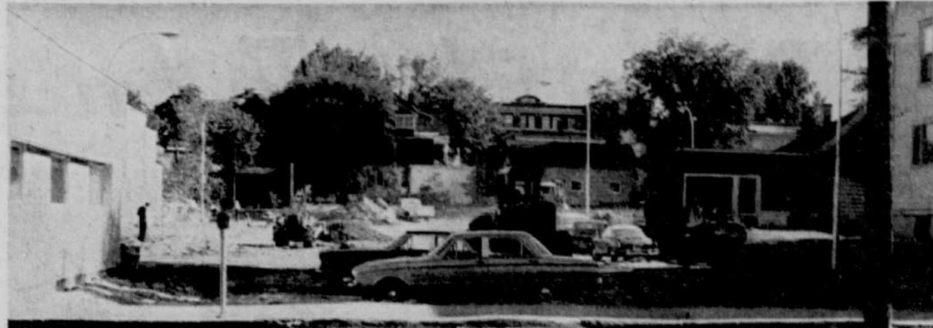
MAGOG'S NEW PARKING LOT — Work is in full swing at Magog where a new municipal parking lot is being built on Main Street West. The area is scheduled for completion by mid-September. (Record photo by Charles Catchpaugh)
