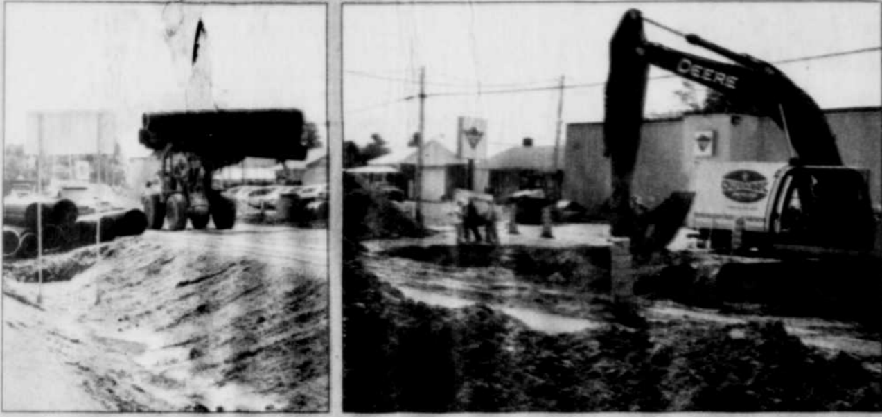
The construction on Hwy 148 outside of Shawville will continue for at least another month. Until then, drivers will have to be patient until the culverts are replaced and the road is raised and repaved.
