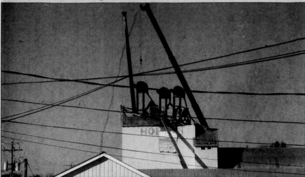
Cranes began the demolition procedure of removing the burnt out elevator of H.I. Hobbs Mill on Tuesday, Nov. 18.
