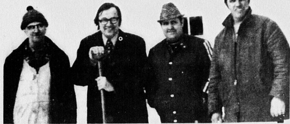
Mayor Claude Pilon of Huntingdon turned the first sod of the Town's new civic centre and police and fire station Monday morning. Left to right in the photo: Lucien Loiselle, excavation contractor; Mayor Pilon and shovel; Ald. Gerald Brisebois, Town Foreman Philibert Langevin.
