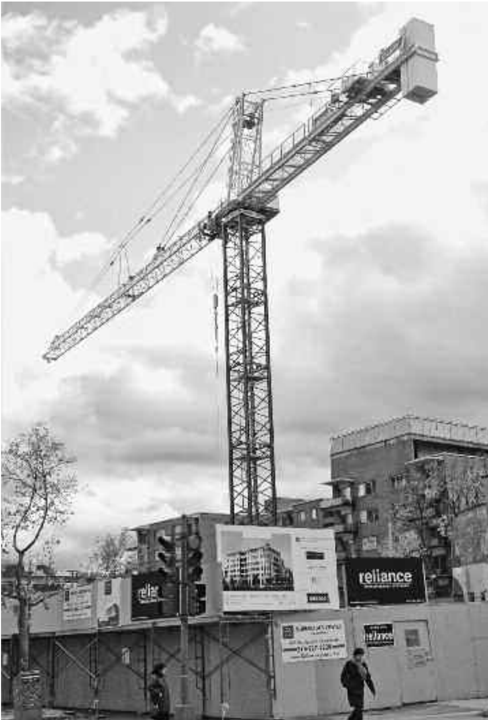
A view of a massive crane looming over the construction site at 1250 Greene Ave., November 11.
