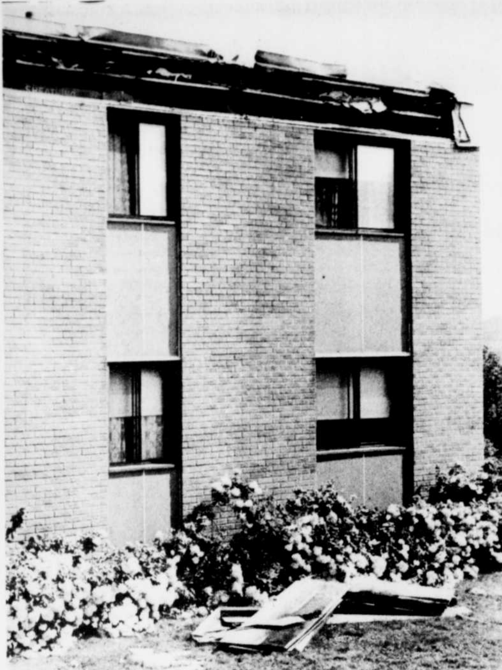
Approximately $25,000 damage was caused by a fire in the roof of this residence at 430 Beaumont Street in Cowansville Monday night. (Record Photo by Nelson Wyatt)
