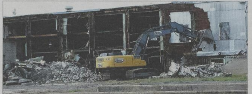
The Town of Huntingdon began demolition of a portion of the old Cleyn & Tinker factory on Route 202 on Wednesday, September 3. The portion of the building being torn down had been contaminated several decades ago and needed to be demolished in order to decontaminate.
