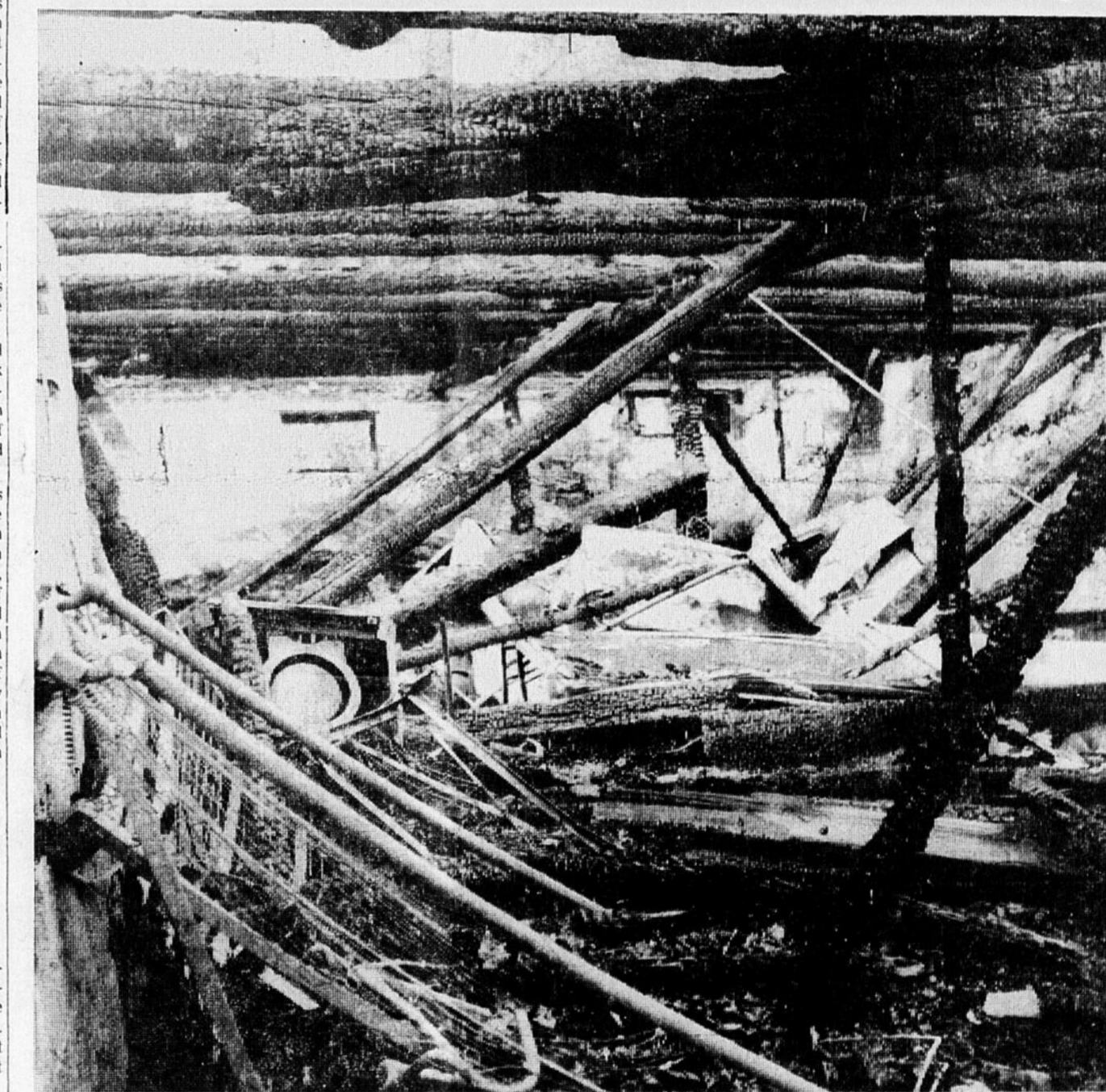
This particular barn was destroyed when fire swept through it early Sunday morning. Situated on Poirier's Hill near Herdman border crossing the structure was a complete loss.
