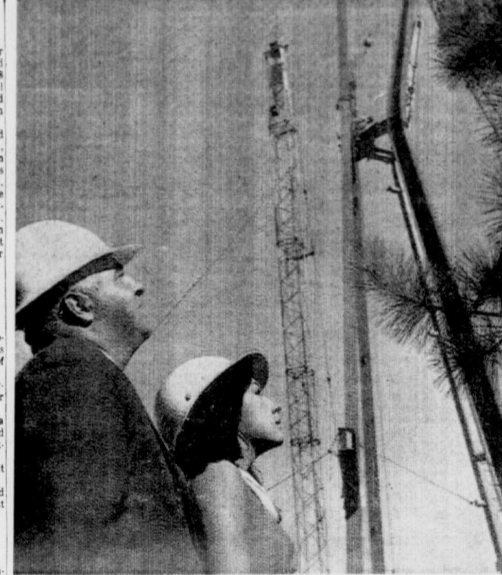
RISING TEPEE — Iroquois chief Andrew Delisle, commissioner general of the Indians of Canada Pavilion at Expo 67, and Diana Diabo, both from the Caughnawaga reserve near Montreal, watch one of the gigantic steel beams being placed on the pavilion which is in the form of a wigwam and will exhibit the culture and art of the Indian. (CP Wirephoto)
