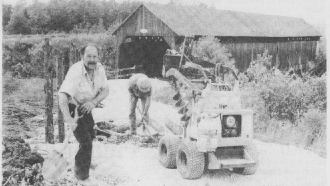
Alain Coulombe and André Pettigrew were hard at work Saturday doing their part to give the John Cook bridge a new lease on life. RECORD PHOTO: PERRY BEATON
