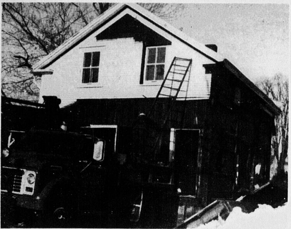
A town crew made short work of this house that was ordered demolished to make room for expansion plans for a new civic building in Huntingdon. Destruction of the old Prince Street house started Thursday morning and by the same afternoon a pile of rubble was all that remained.
