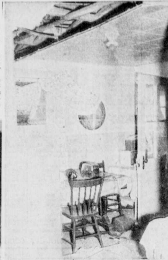
FLOORS AND WALLS TORN OUT — The interior of the Rudolph Tropper home after the propane gas explosion yesterday morning. (Record photo by Studio Eclair)
