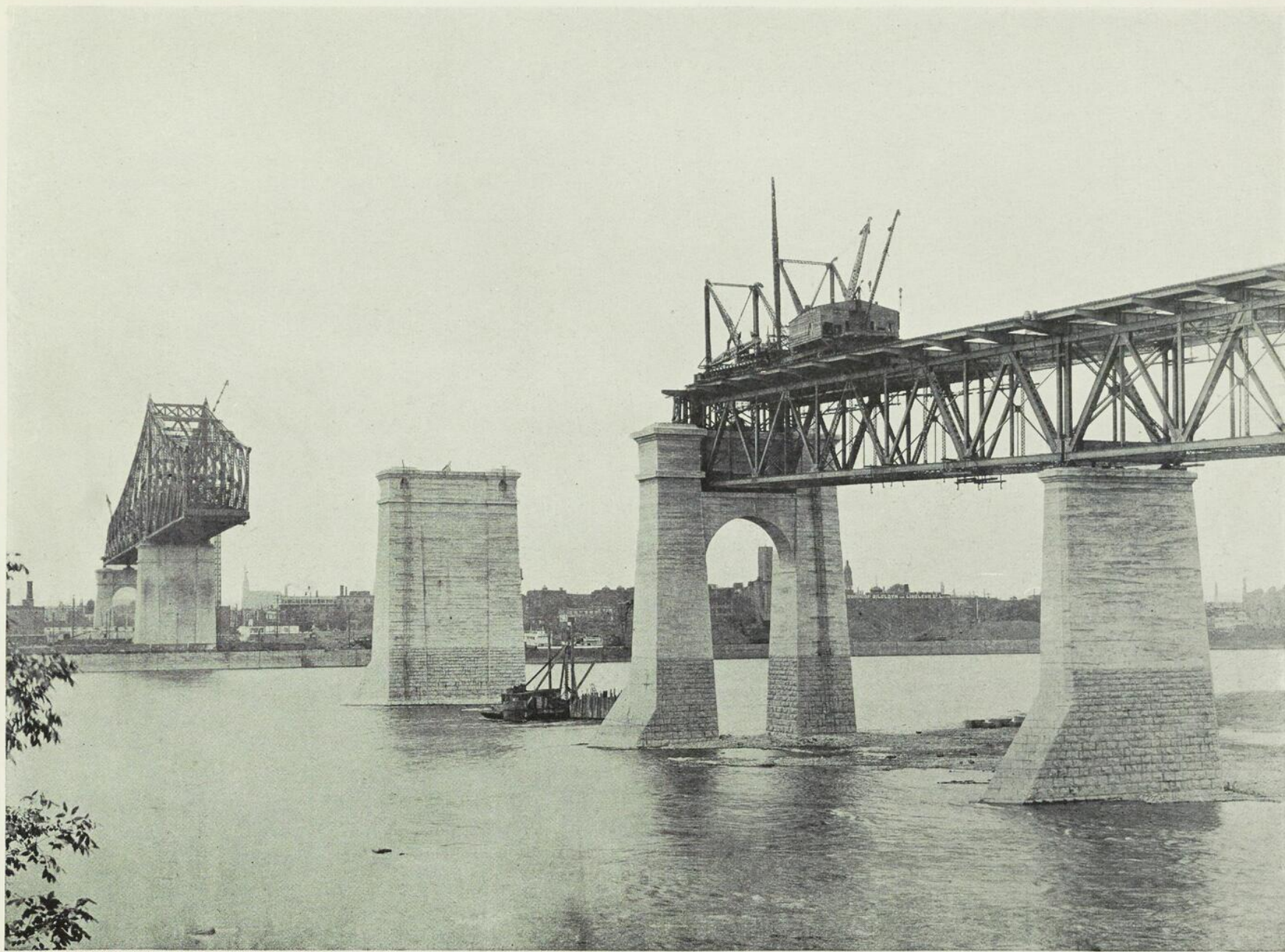
Figure 15. —SOUTH APPROACH COMPLETED. TRAVELLER FOR ERECTION OF FALSEWORK BEING SET UP, AND TEMPORARY PIERS UNDER CONSTRUCTION. 29
