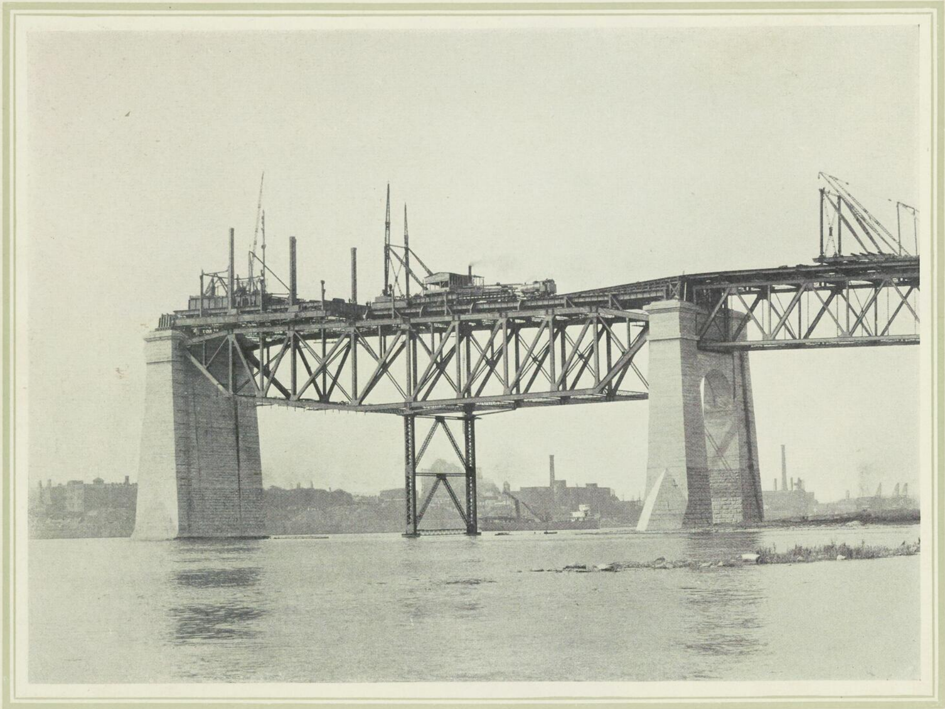
Figure 20. —ERECTING CHORDS AND FLOOR SYSTEM OF SOUTH ANCHOR ARM, AND MAIN TRAVELLER.
