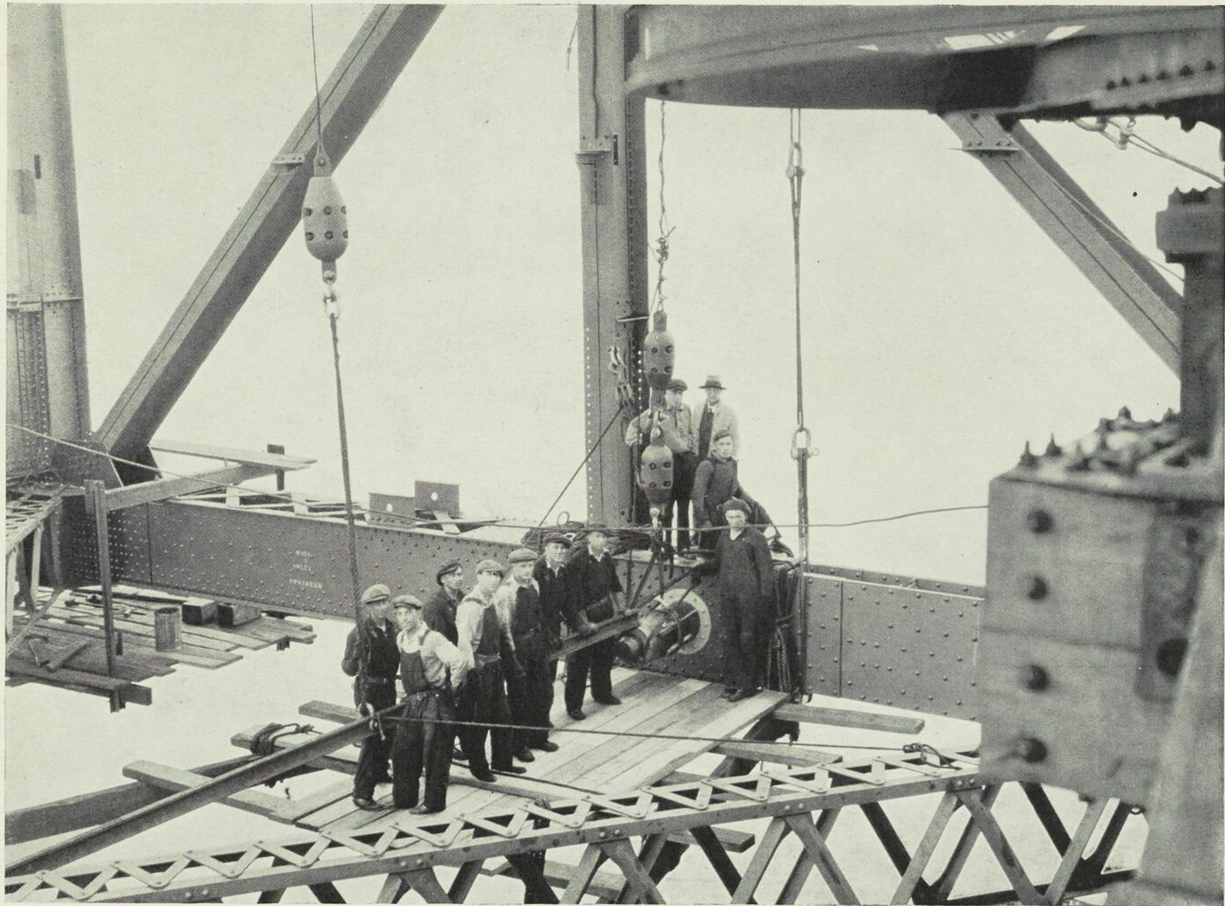
Figure 31. —DRIVING PIN IN BOTTOM CHORD AT CENTRE OF SPAN ON DAY OF CLOSURE.
