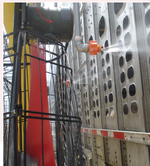
Combined water sprinkling and ventilation system. Source: Sherbrooke Research and Development Centre, AAFC
