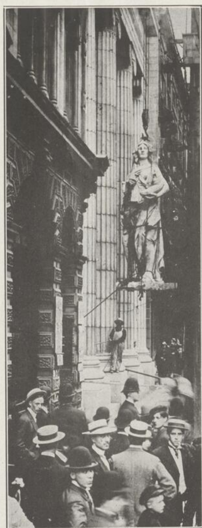
MODERNIZING ST. JAMES STREET, MONTREAL—Elevating one of the four huge marble statues, emblematic of the industries of Canada, to the top of the portico of the new Royal Bank. The immense size of the statue may be best judged by comparing it with the man below.
