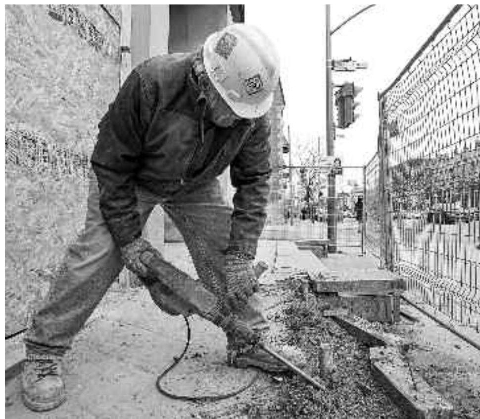
Construction foreman Yves Raymond of Emcon Construction uses a hydraulic drill-hammer to remove a section of the entrance ramp at the former post office at the corners of Sherbrooke and Prince Albert, March 27. The vacated building is being prepared for its new occupant, Lululemon Athletica.
