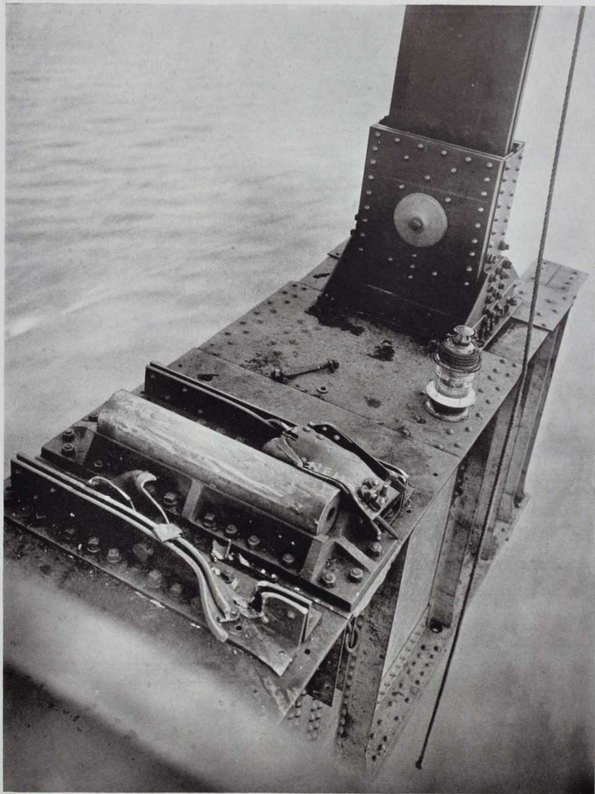
65—Condition of lower shoe and carrying girder after the loss of the suspended span
