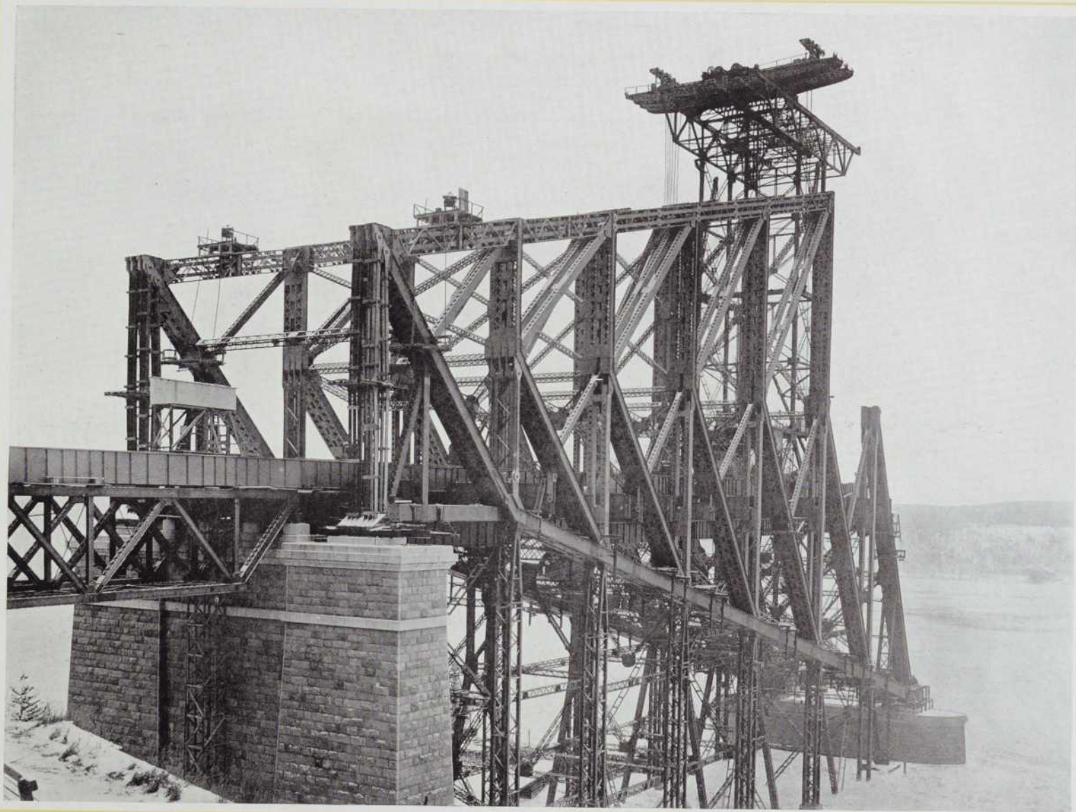
26—Condition of the North anchor arm at the close of the season of 1914
