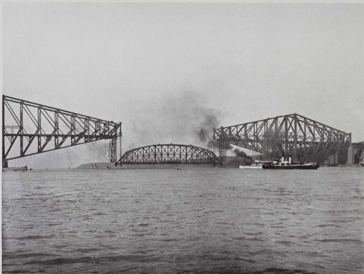
61—September 11, 1916, 10.40 a.m. Just before the loss of the suspended span
