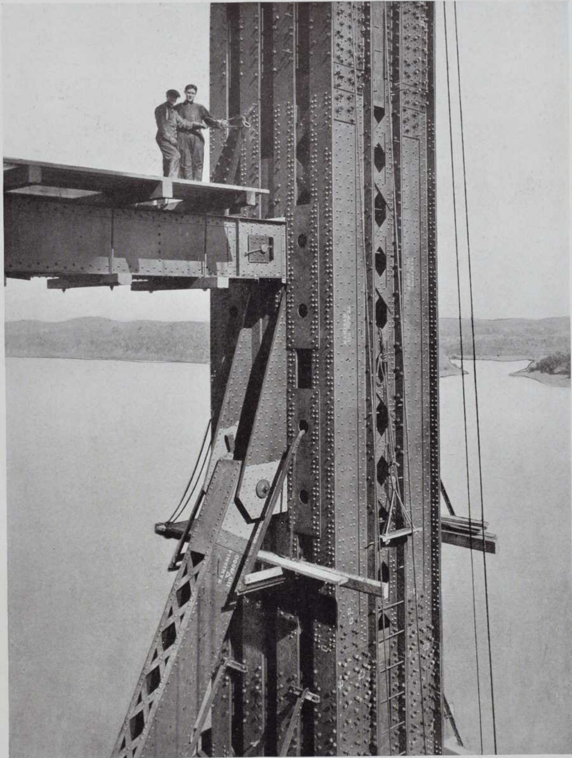
27—Connection of web members at the centre of the large post over the main pier
