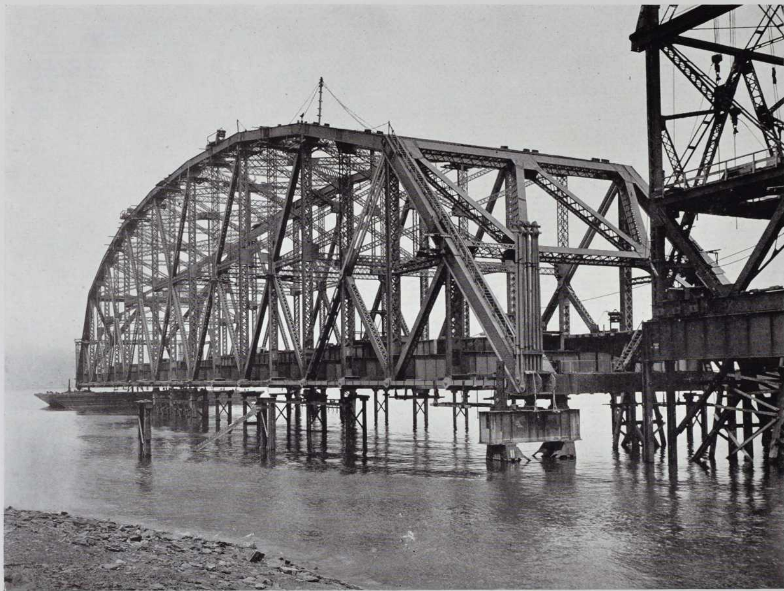
49—The falsework removed with the suspended span resting on the end supports
