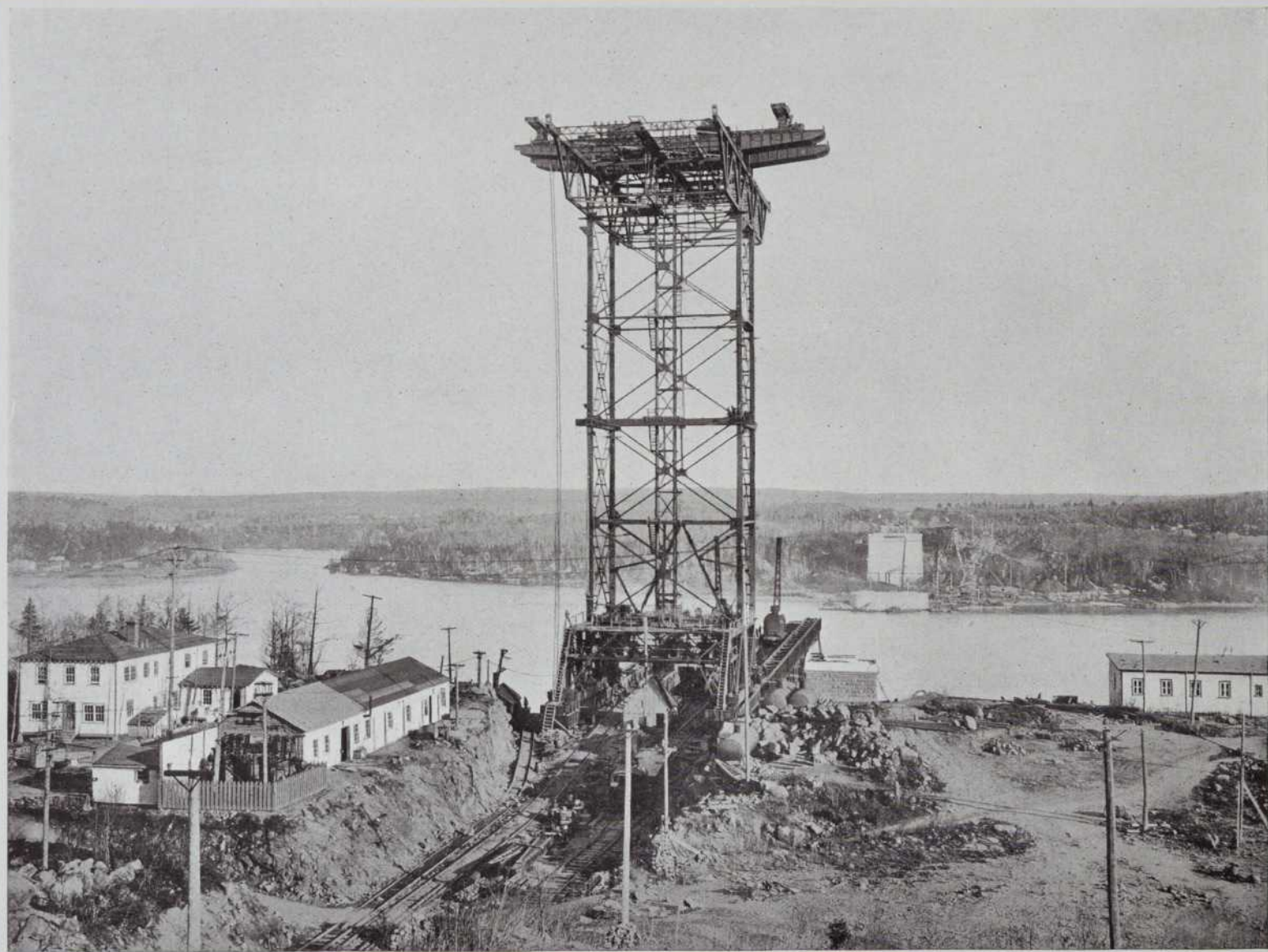
15—The North Shore traveller erected being equipped, also showing the office building and power house to the left
