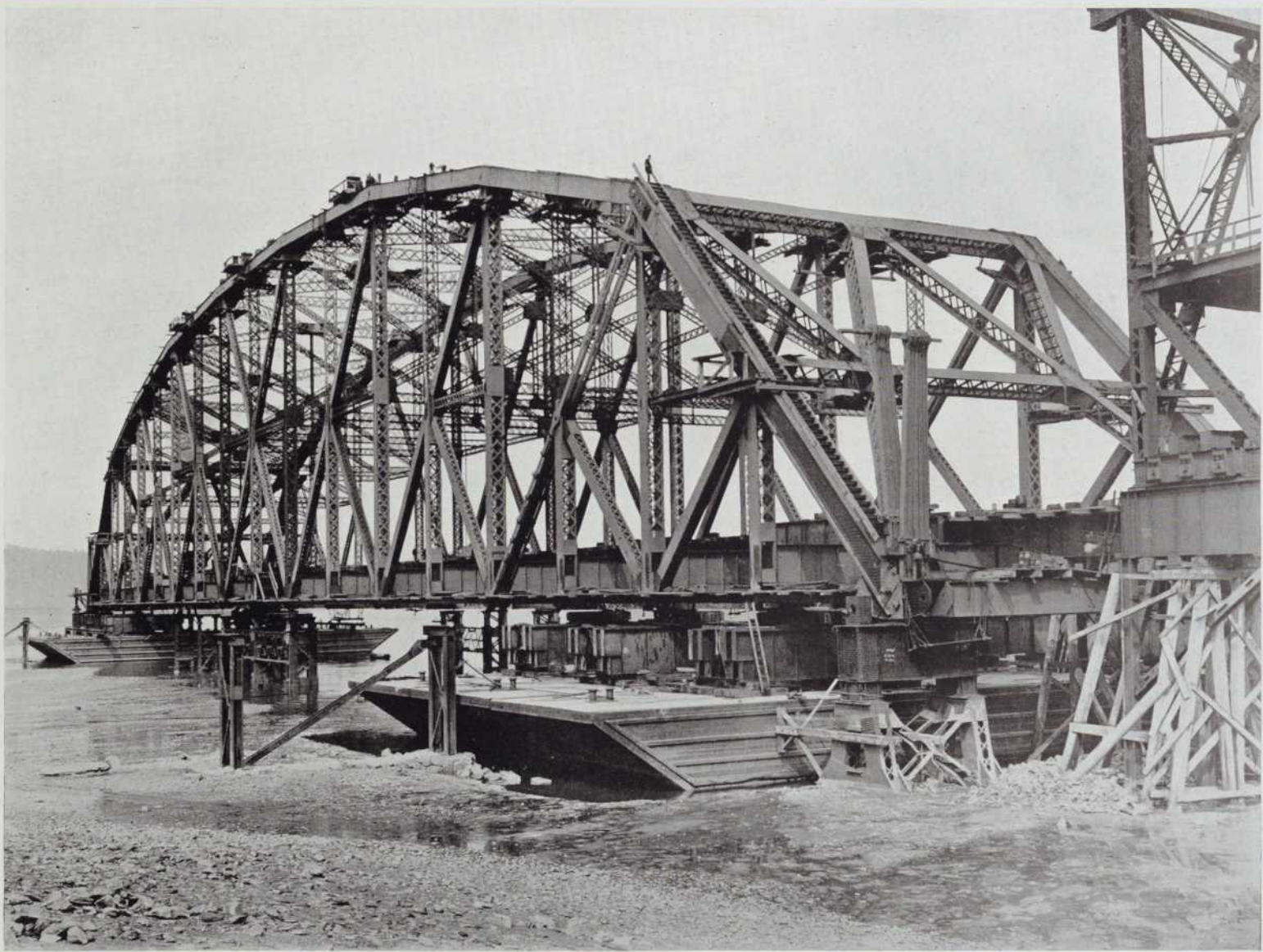
50—The suspended span resting on the end supports at Sillery. The falsework removed and the scows blocked under ready for floating
