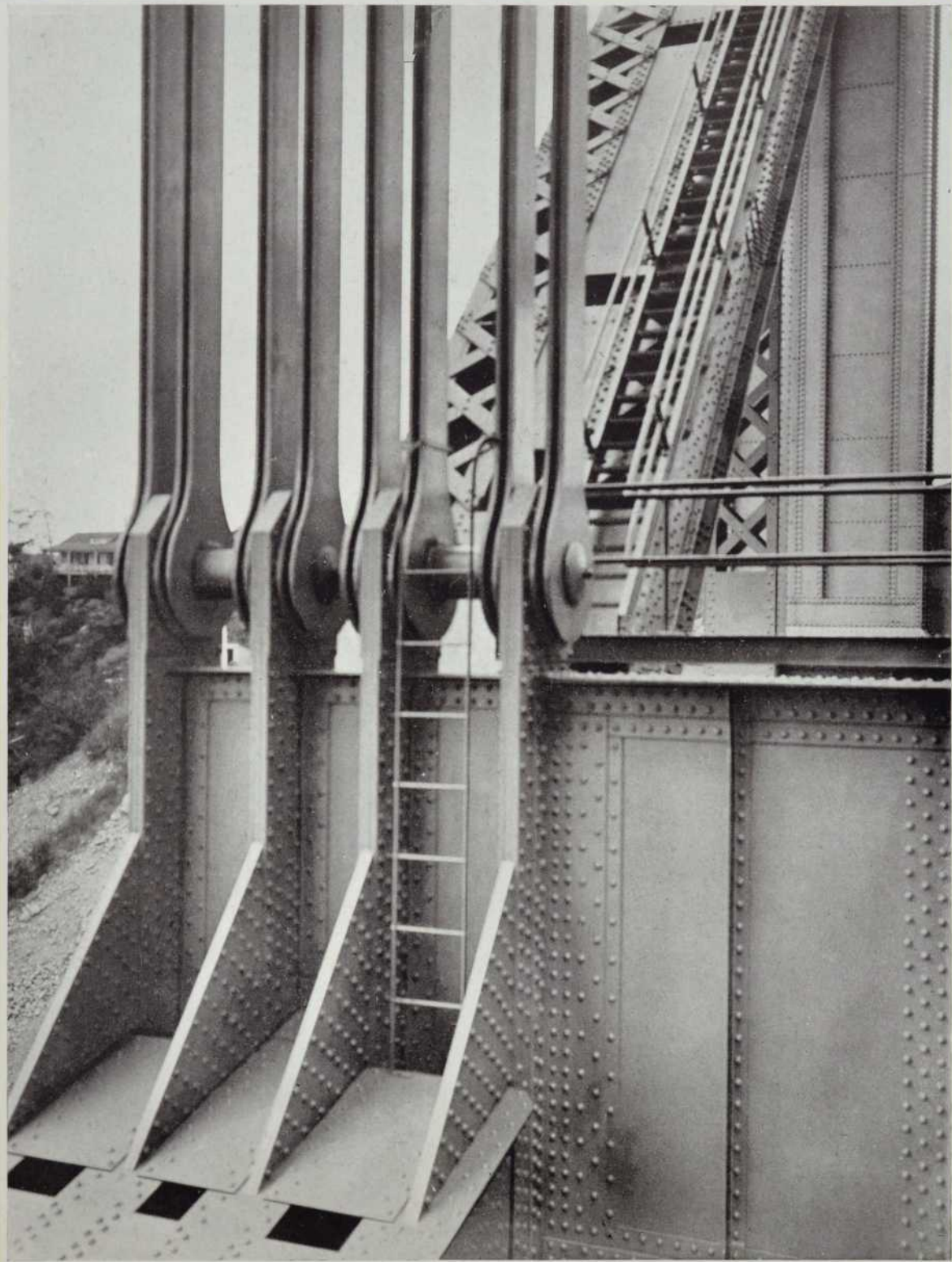
75—Detail at AL2, showing the floorbeam connection to the outer end of the Anchor Arm bottom chord
