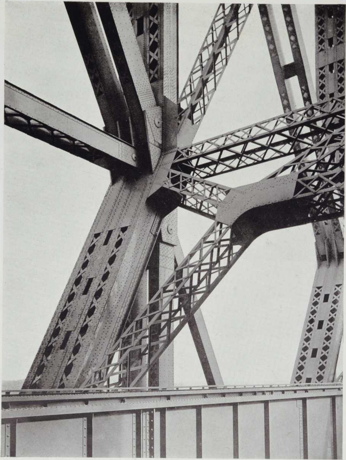
74—Detail at CM 14. The middle panel point of the cantilever Arm adjacent to the Main Post.
