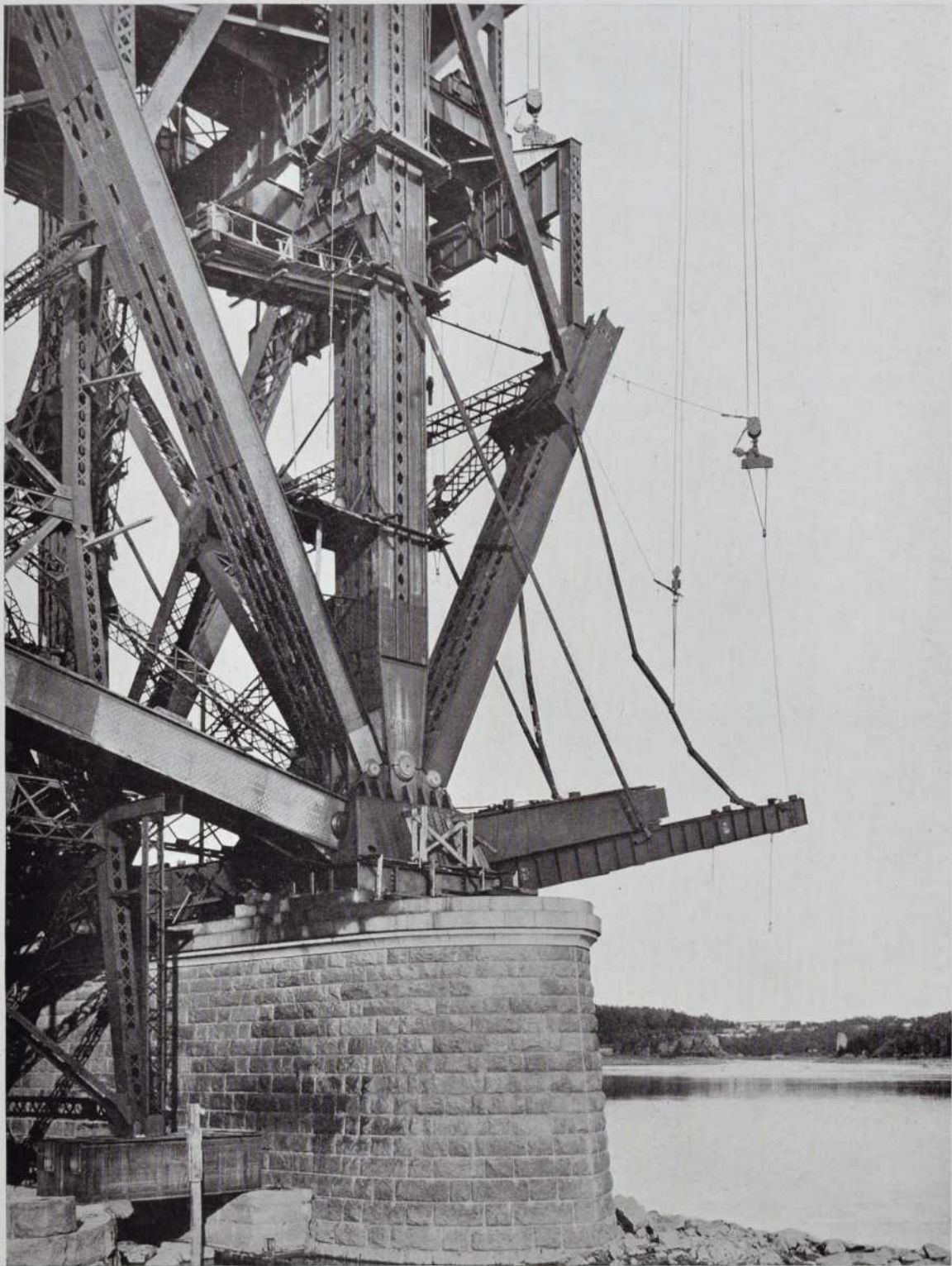
31—Starting the erection of the North Shore cantilever arm, showing the supporting platform in place carrying the first sections of the lower chord
